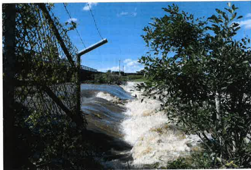
Fig 10 Concrete weir obstructing flow
