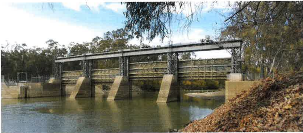
Fig 15 Stevens Vertical Lift Bulkhead Weir
